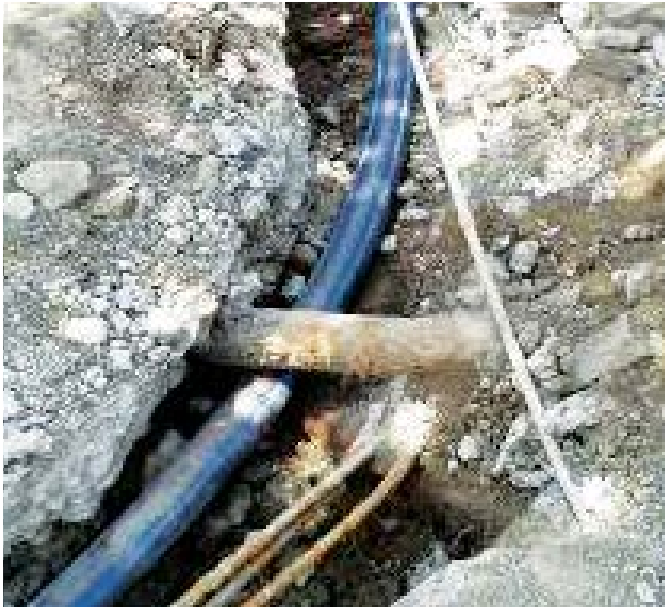
Fig 8: Concrete overburden on utility lines difficult to handle by open trench
